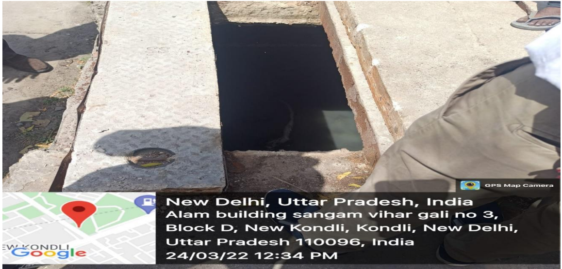
Figure 3: Free- Flowing Wastewater observed at 100 m downstream of Kondli diversion section
